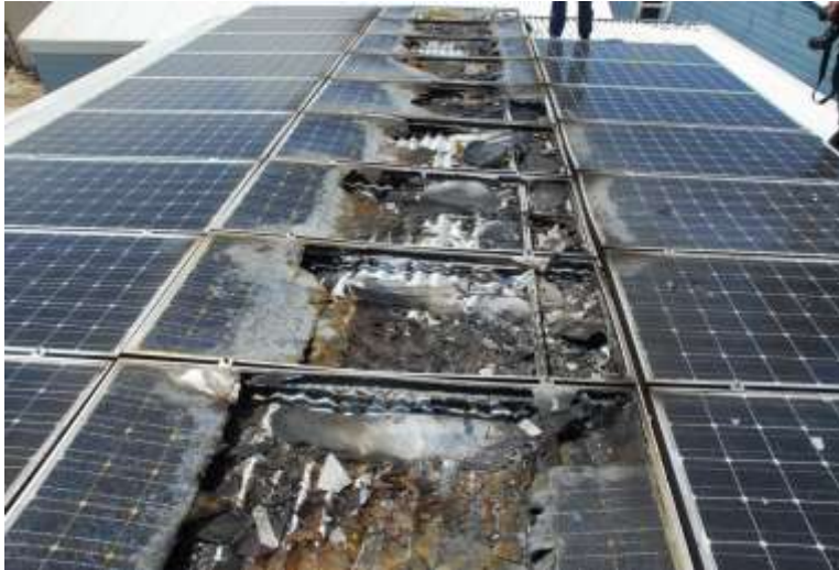
DC system with panel failure which caused arcing and subsequent fire in SA Nov 2011.
